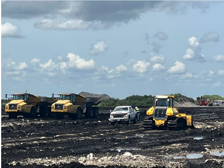
Everglades Agricultural Area Reservoir, Construction of Inflow-Outflow and Seepage Canals underway, APR 2023
